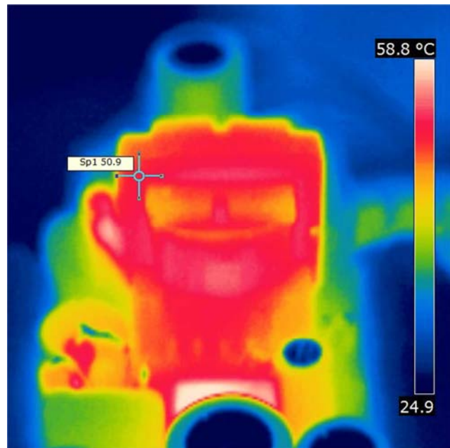
Figure 25 – SP1 – Transformer (T1).
