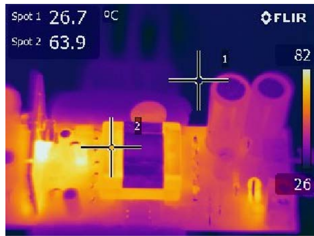
Figure 32 – 230 V VAC, Full Load. Spot 2: Transformer (T1): 63.9 °C.
